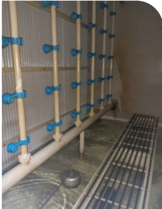
Directly after cleaning
